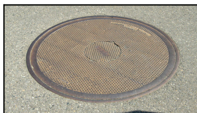
Electrical or Communication Vaults
