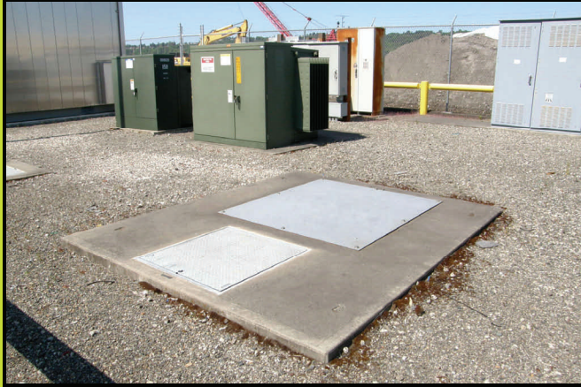
Electrical or Communication Vaults on our terminals
