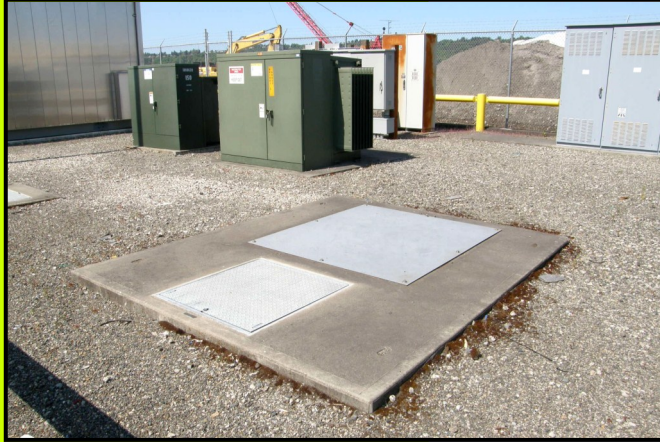
Electrical or Communication Vaults on our terminals
